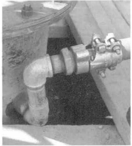
Figure 15.24. In the pressurization method, the eductor and air line are placed in the well and then the casing is capped. (Bergerson-Caswell, Inc.)
