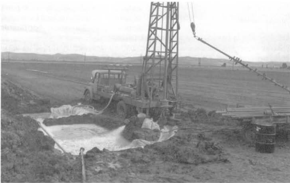
Figure 10.12. Drilling fluid from the borehole flows into the larger pit where the cuttings settle out. The fluid then flows into the second pit through a constricted opening. The mud pump on the rig withdraws drilling fluid from this pit to inject down the drill rods to the bit. This Italian driller has lined the drilling fluid pits with polyethylene film to reduce fluid loss into the ground. Note the homemade hole cleaner or scratcher the driller uses to keep the borehole open during drilling.
