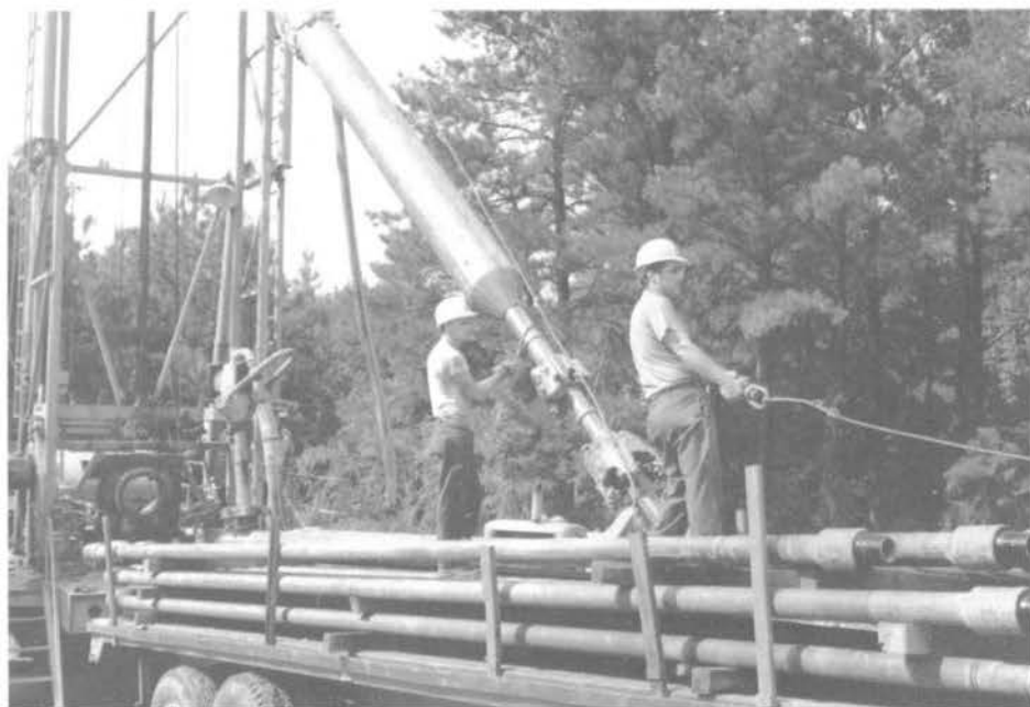
Figure 10.17. Heavy collars added to the drill string above the bit help keep the borehole straight.
