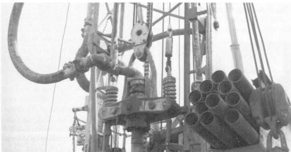
Figure 10.21. The upper end of the kelly connects to a swivel suspended from a traveling block in the mast. (E. H. Renner & Sons, Inc.)
