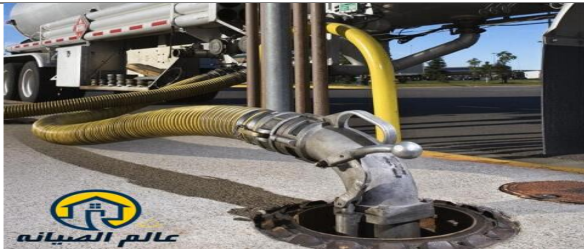
Figure 7.5: Handle to Prevent Contact with Sludge; Reference Image
