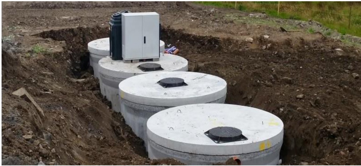
Figure 7.3: Septic Tank Riser
