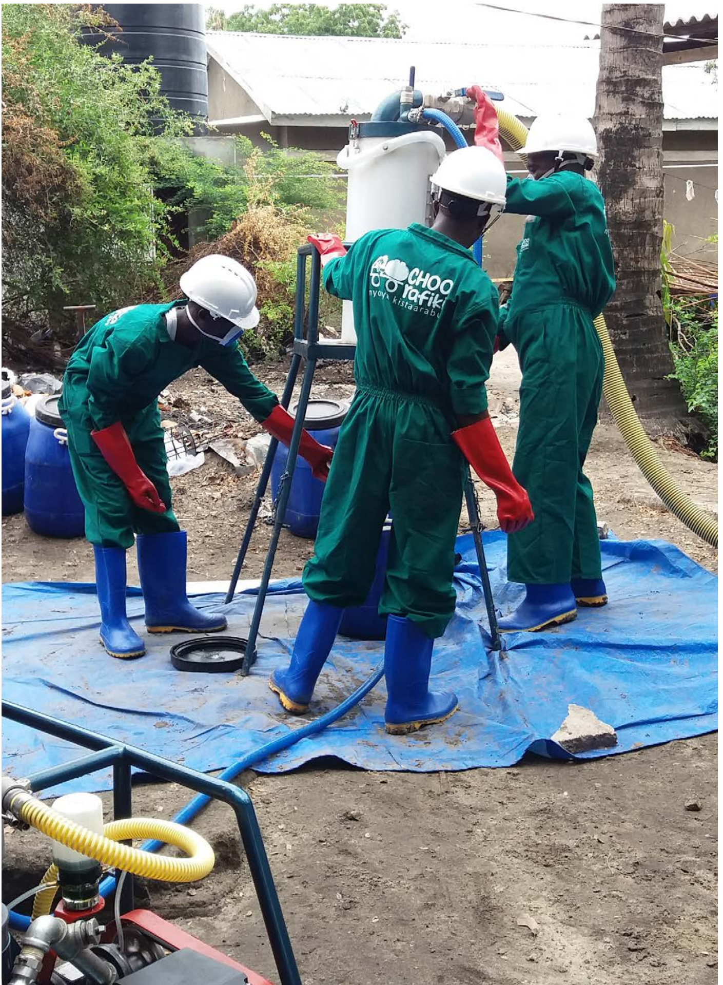
Figure 2 Small-scale emptying services with eVac and motorised tricycle
