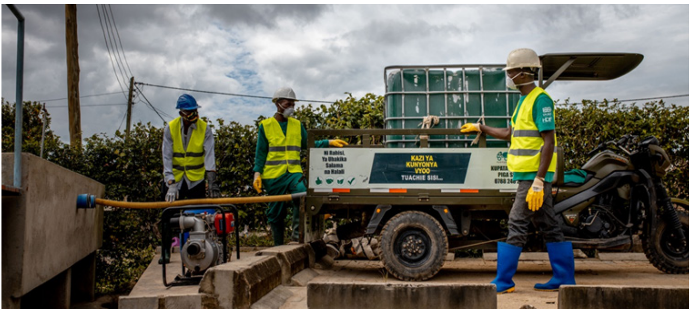
Figure 54 Service providers discharging sludge into Mburahati - Ubungo FSTP
