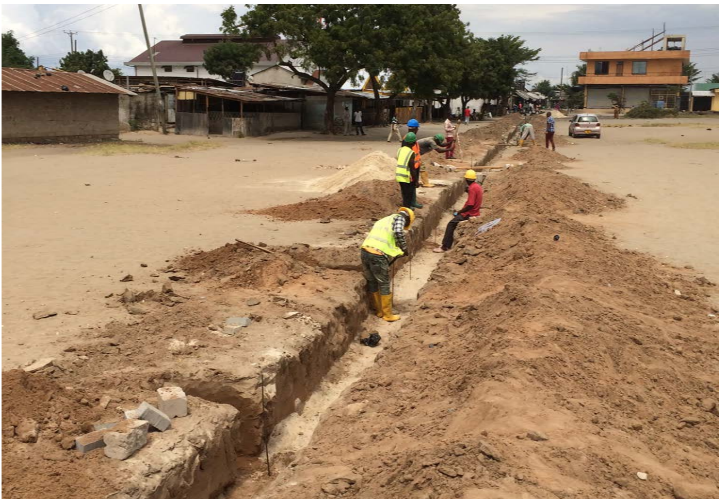
Figure 33 Implementation of a water distribution system - reusing the FSTP effluent for landscape irrigation in Mburahati
