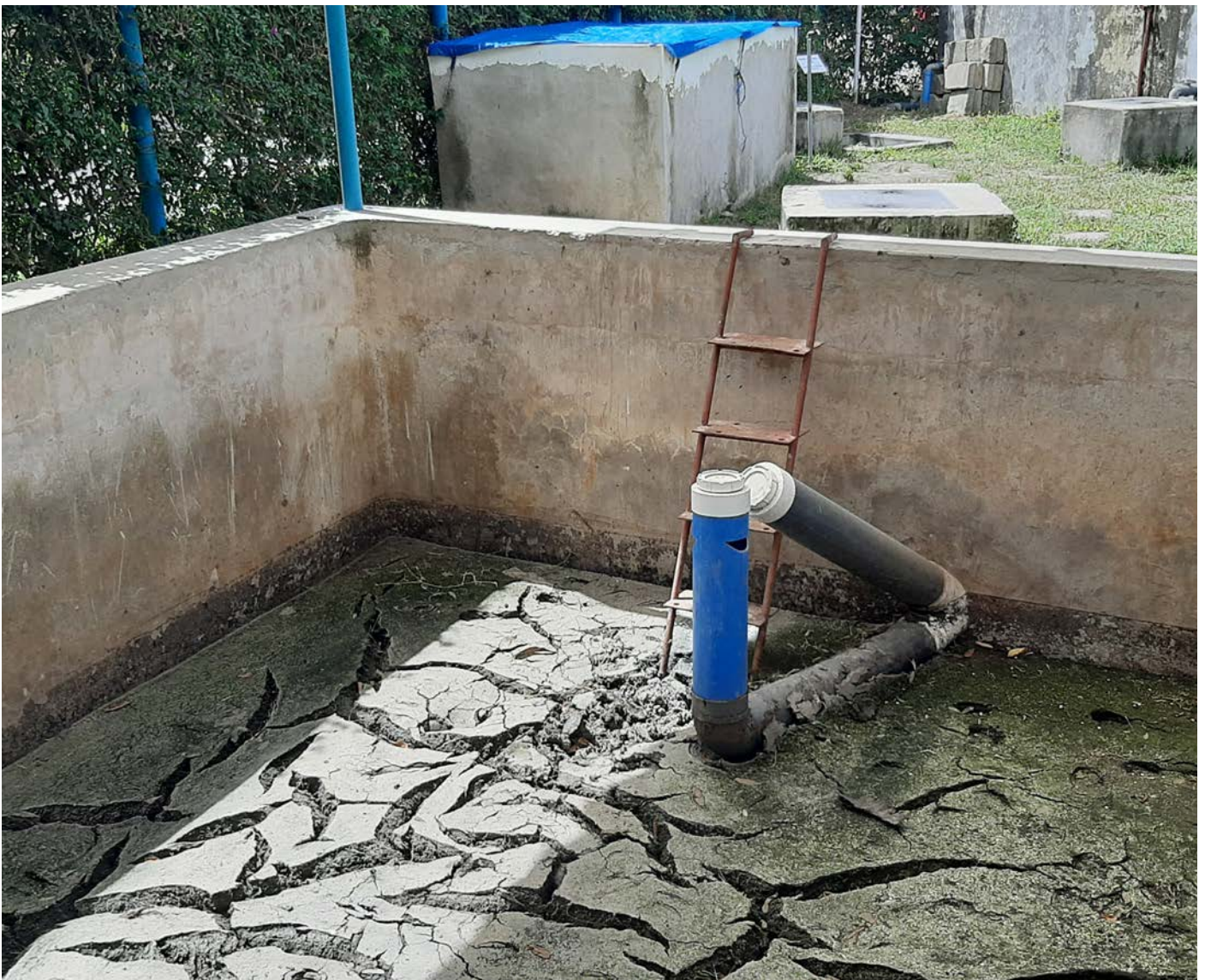
Figure 42 Unplanted drying bed at Mburahati-Ubungo FSTP
