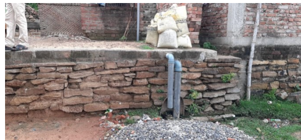
Figure 4: Septic Tank Connected to Open Drain (CSE/Chirag Patel, 2021).
