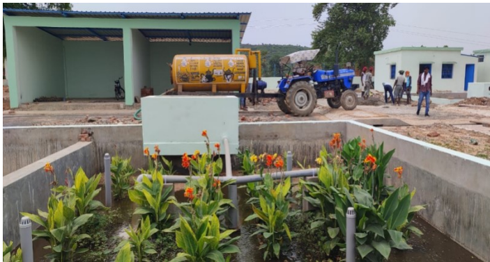
Figure 8: Discharging of FS at Planted Drying Bed (CSE/Shantanu, 2021).
