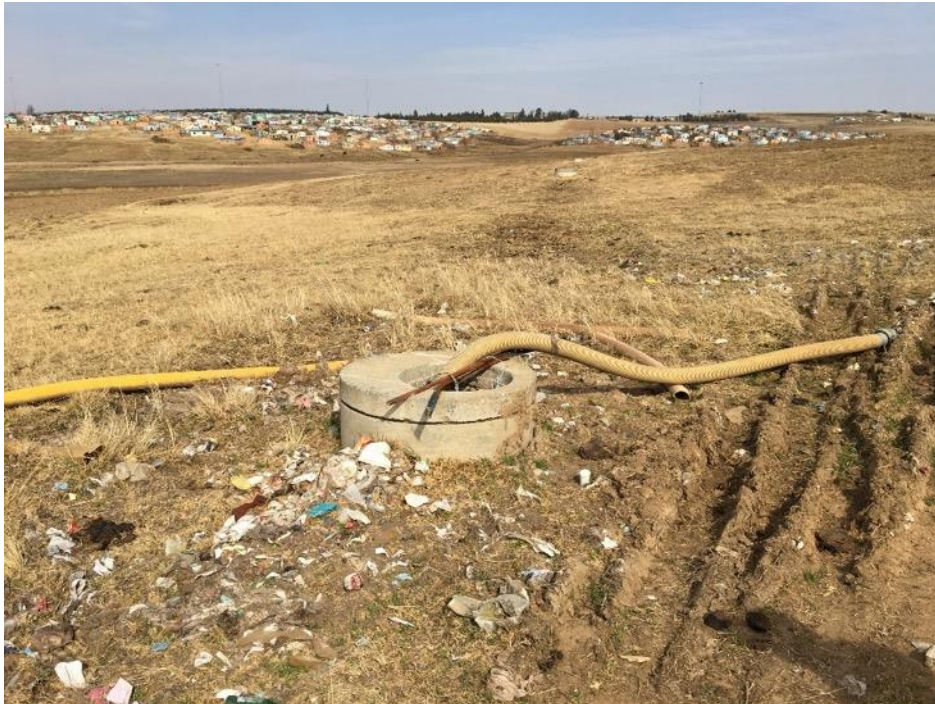
Figure 10: Tanker discharge point at Prentjiesberg WWTW
