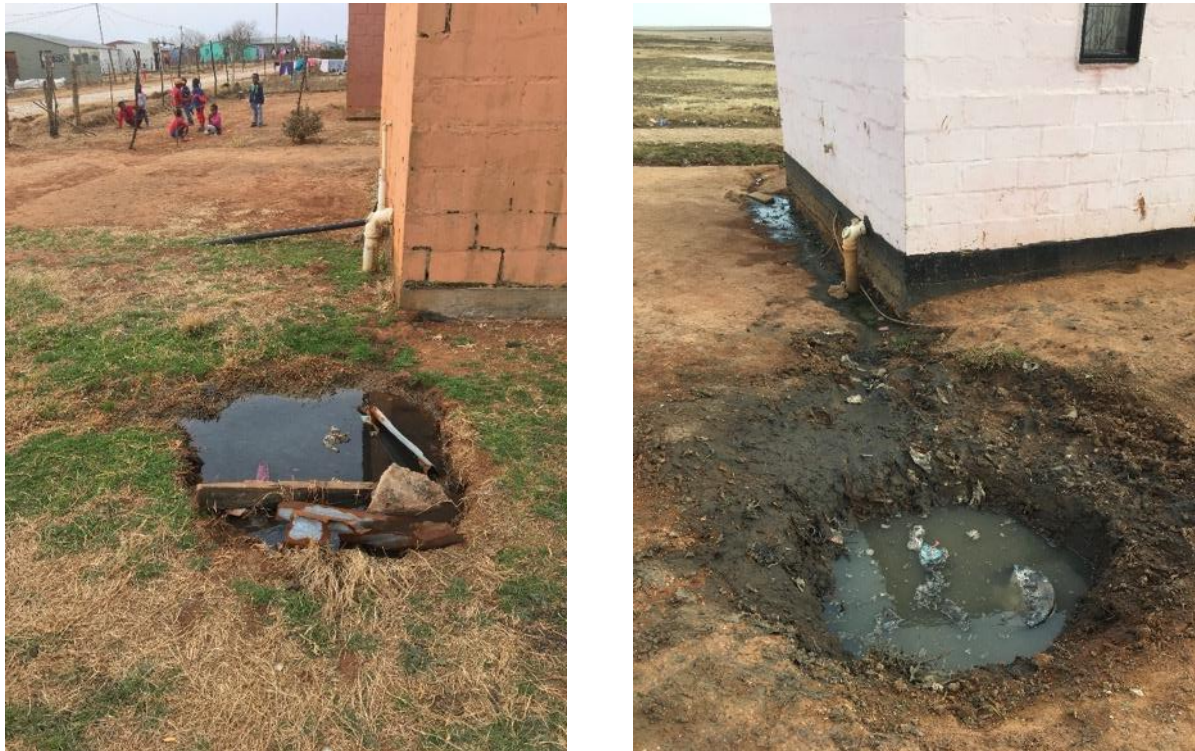
Figure 8: Evidence of full and overflowing containment tanks
