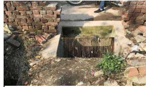
Figure 4: Interception point at Diwani talab mandi for open drains (Source: Harsh/CSE/2021).
