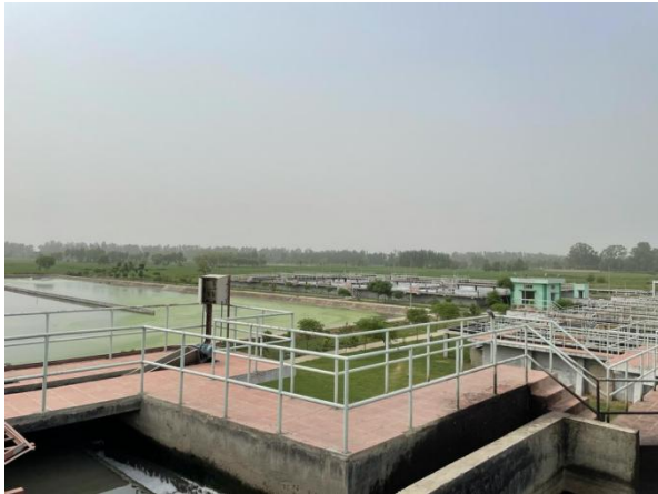
Figure 9: STP (capacity 24 MLD) in Bijnor City. (Source: Harsh/CSE/2021).
