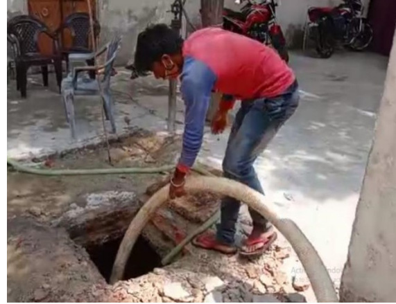
Figure 11: Emptying of a fully lined tank by desludger (Aamir/CSE/2021).
