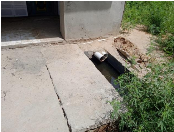
Figure 8: A Community toilet with a septic tank connected to open drain. (Aamir/CSE/2021).
