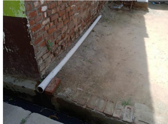
Figure 9: Supernatant flowing into open drain from a septic tank. (Aamir/CSE/2021).
