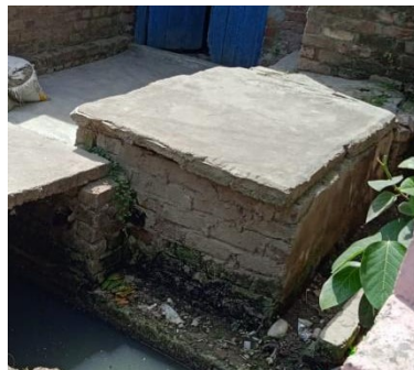
Figure 6: A fully lined tank connected to open drain. (Aamir/CSE/2021).
