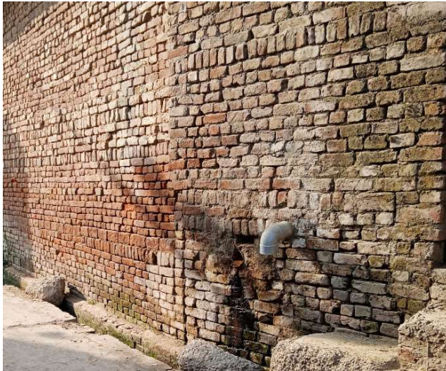
Figure 3: Toilet connected to open drain (Aamir/CSE/2021).
