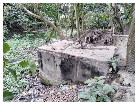
Septic tank directly discharges to a pond, no soak pit
