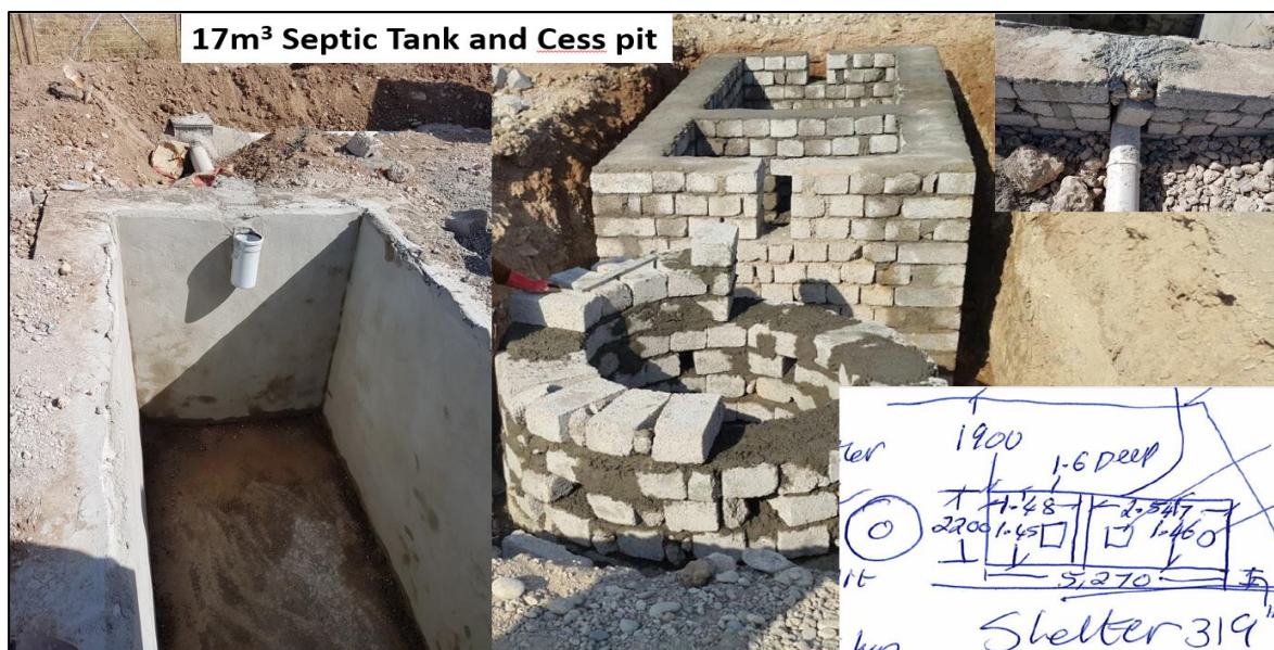
Figure 14: Blockwork septic tank and soak pit, New Zozan, Domiz 1. (Source: UNHCR Duhok, 2019)
