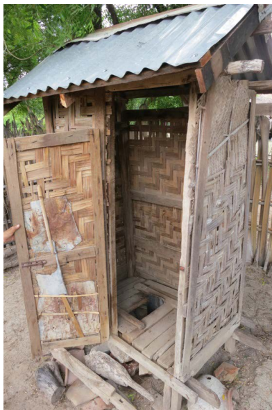
Image 4 - Typical latrine type - Myanmar
