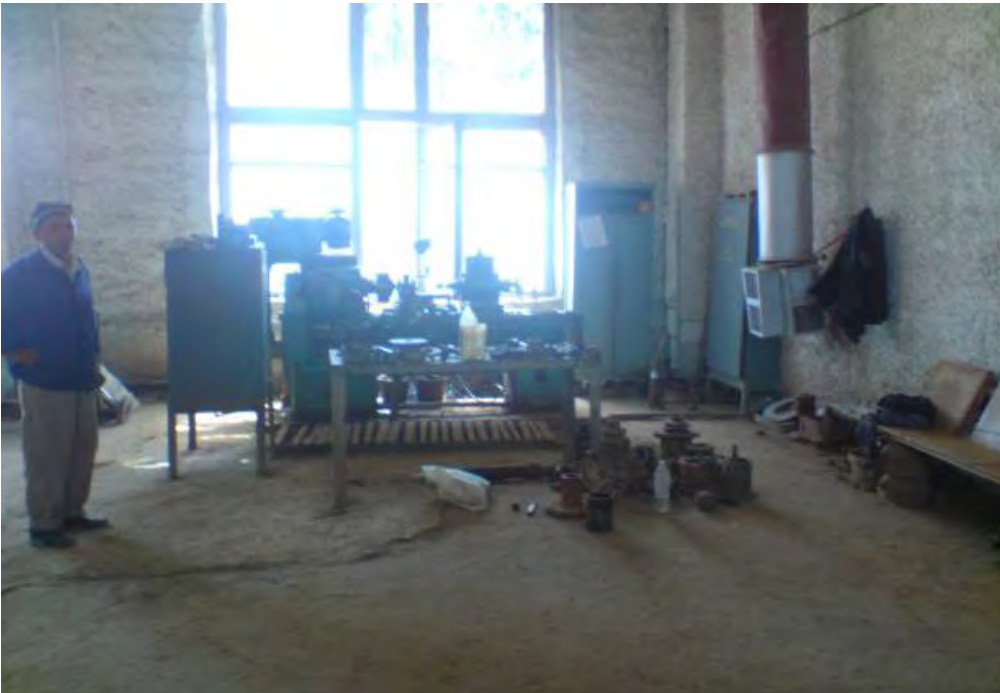
Photo 4. Workshop for repairing of pumps of the Water Distribution Unit “Kurpa”
