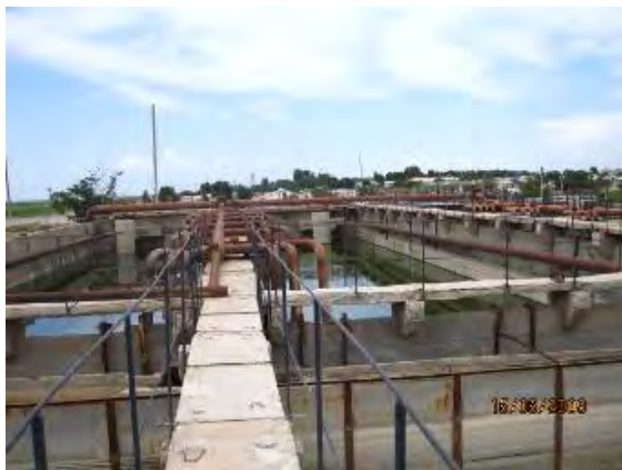
Figure 6. Aeration tanks (25,000 m 3 /day)
