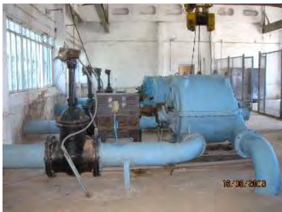
Figure 7. Air blower Compressors
