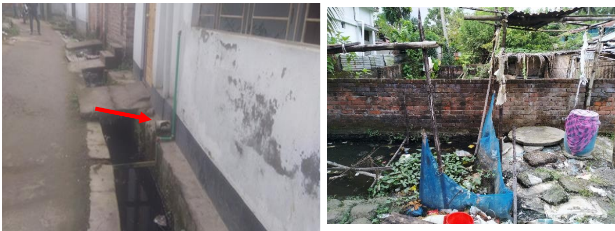
Figure 6 : Containment technologies and their connections in Bagerhat Left: Toilet Pit open to a nearby water body, Right: Toilet pipe connected to open environment
