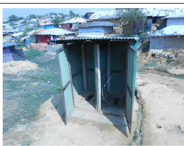
Latrine block in Camp 6 with no hand-washing present
