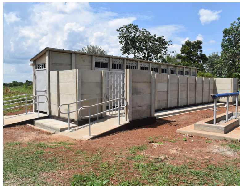
A new block of toilets built at one of Apac Municipality beneficiary institutions, northern Uganda
