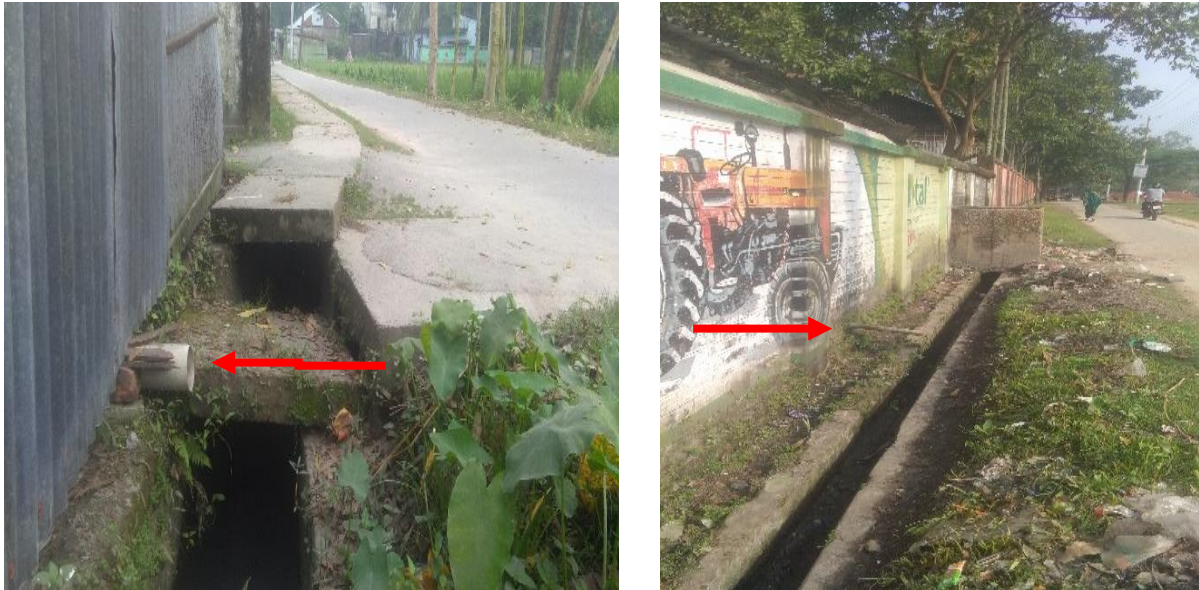
Figure 6: Containment technologies and their connections in Lalmonirhat. Left: Septic tank connected to the nearby water body. Right: Toilet pipe connected to open drain. (Source: Feasibility study 2020-21/DPHE).
