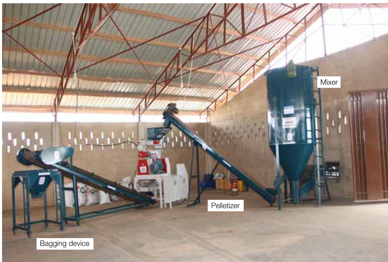
FIGURE 7. PROCESSING EQUIPMENT INSTALLED INDOORS AT THE FORTIFER PLANT IN GHANA.
