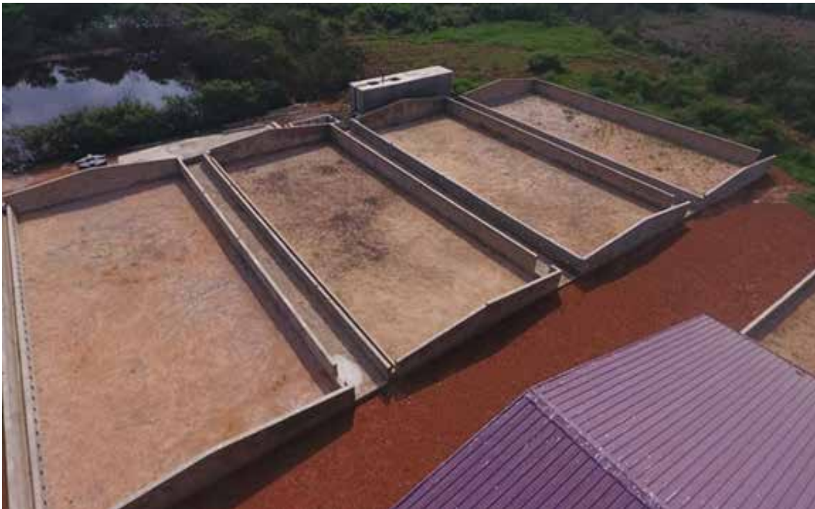
FIGURE 3. AERIAL VIEW OF FOUR DRYING BEDS BEFORE LOADING WITH FS AT THE FORTIFER PRODUCTION PLANT, GREATER ACCRA, GHANA.
