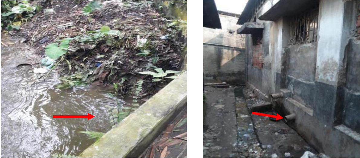
Figure 6: Containment technologies and their connections in Joypurhat. Left: Septic tank connected to the nearby water body. Right: Toilet pipe connected to open drain. (Source: Feasibility study 2020-21/DPHE).
