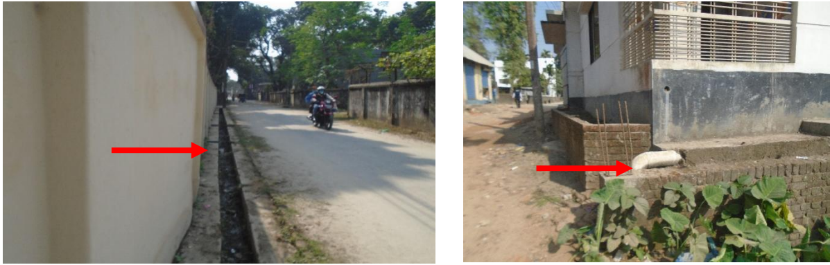
Figure 5: Containment technologies and their connections in Thakurgaon. Left: Septic tank connected to the nearby water body. Right: Toilet pipe connected to open drain. (Source: Feasibility study 2020-21/DPHE).
