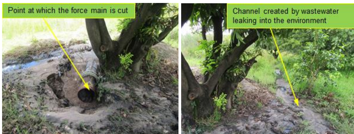
Figure 4: Vandalised force main at Industrial SPS resulting in wastewater leaking into the environment.
