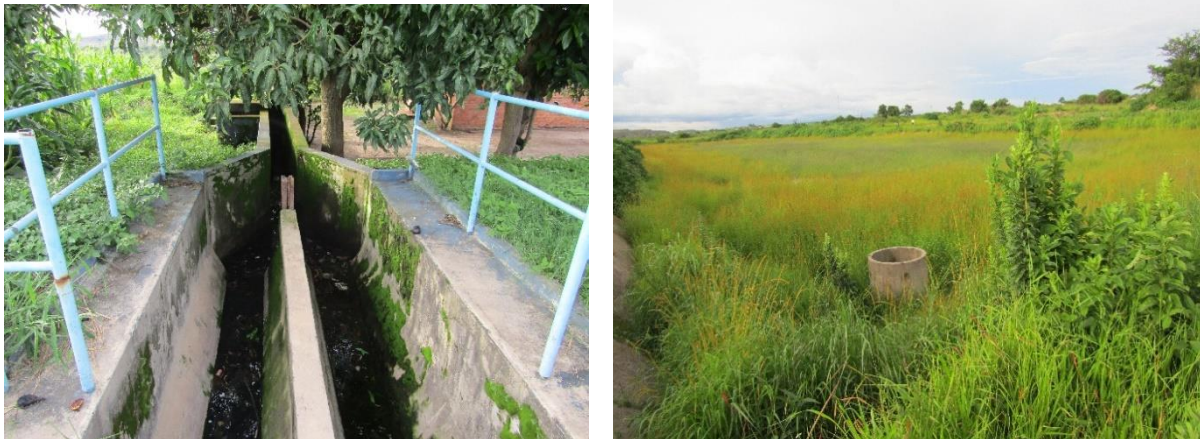
Figure 5: Evidence of low wastewater volumes reaching the treatment plants (LHS: A dry section of the channel for the Lulamba Sewage Ponds; RHS: Dry maturation pond at the Lulamba WWTP that has not received wastewater the past six years.
