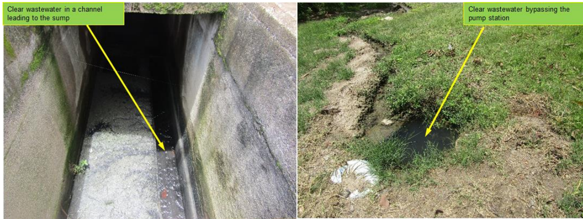
Figure 3: Clear wastewater devoid of solids arriving at the Industrial Sewage Pump Station.
