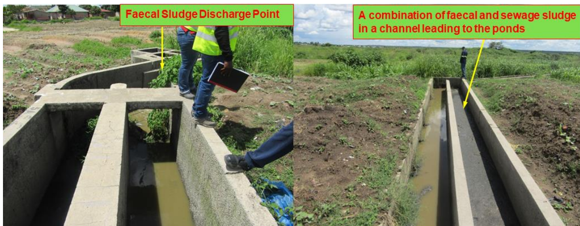
Figure 6: The faecal sludge discharge point on the raw wastewater channel leading to the Chiwempala Ponds.
