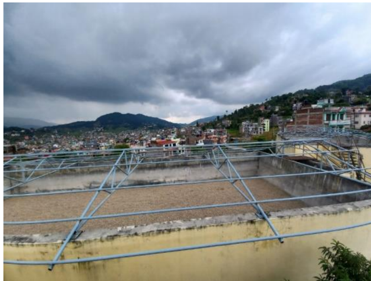
Figure 14: Overview of slow sand filter unit in water supply system developed under KVIWSP.
