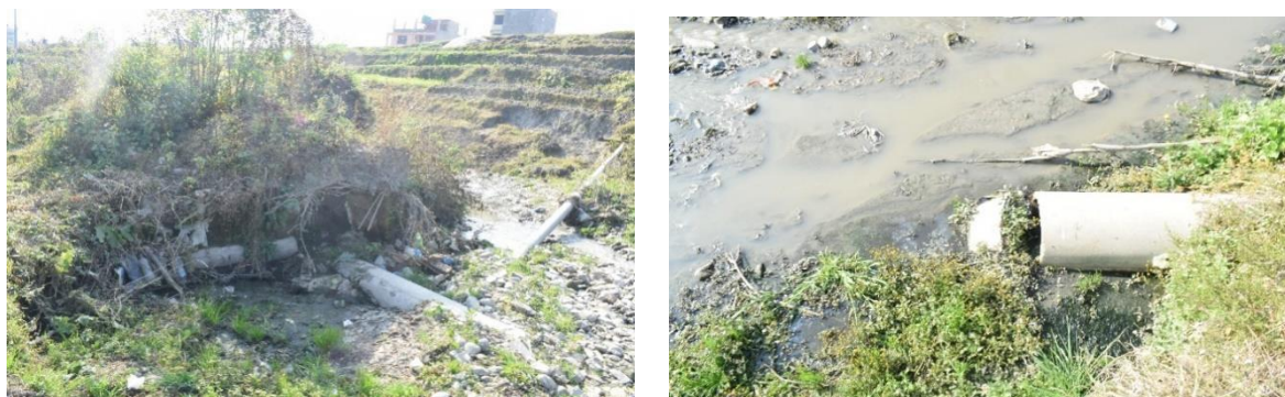
Figure 2: Damaged and disconnected river crossings for sewer networks.
