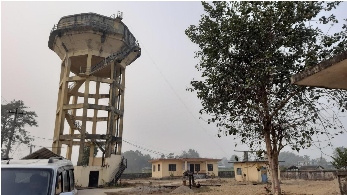
Figure 14: Overhead Tank for Piped Drinking Water System in Harion Municipality
