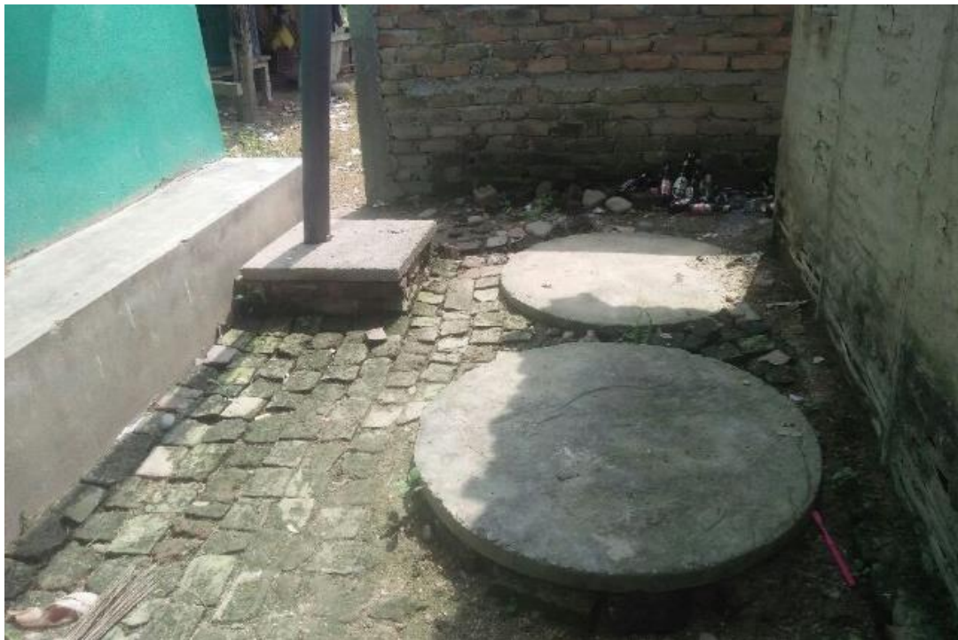
Figure 5: Inappropriate design of the twin pits, where the distance between two pits is less than 1 m.
