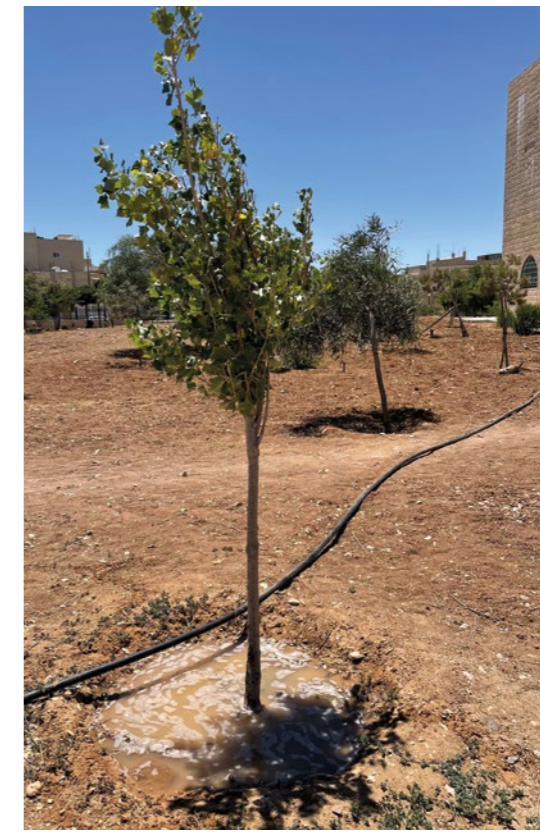
← The greywater recycling system at the Ja'far ibn Abi Talib mosque in Mazar collects water from ablution facilities (left) and treats it so that it can be used to water the gardens (right) and for outdoor cleaning
