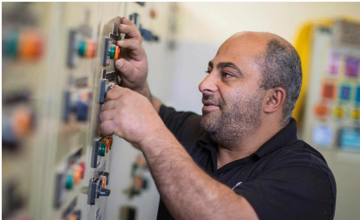
← Operator at the Fuheis wastewater treatment plant
