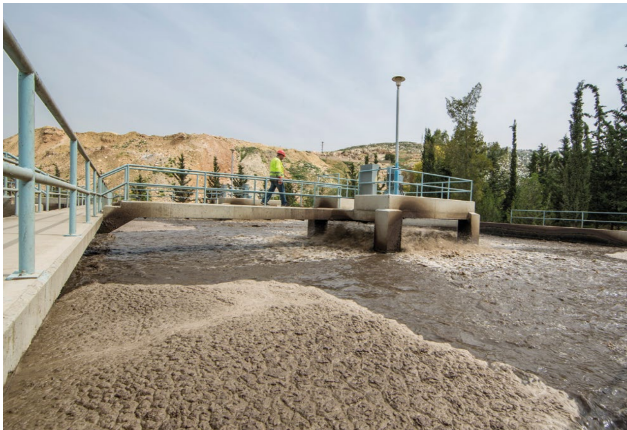
← Fuheis wastewater treatment plant
