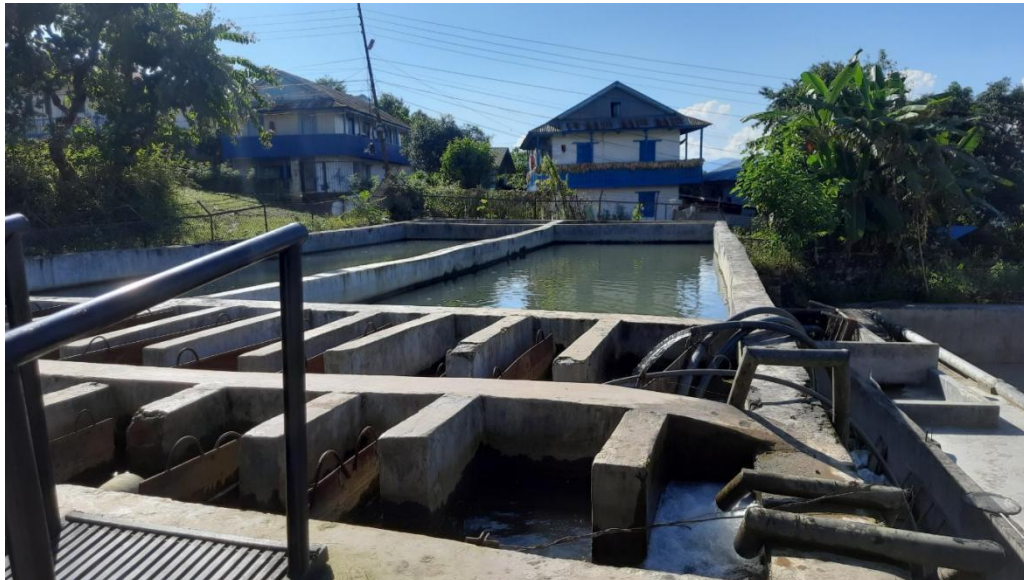
Figure 13: Conventional Water Treatment Plant available in the Municipality.
