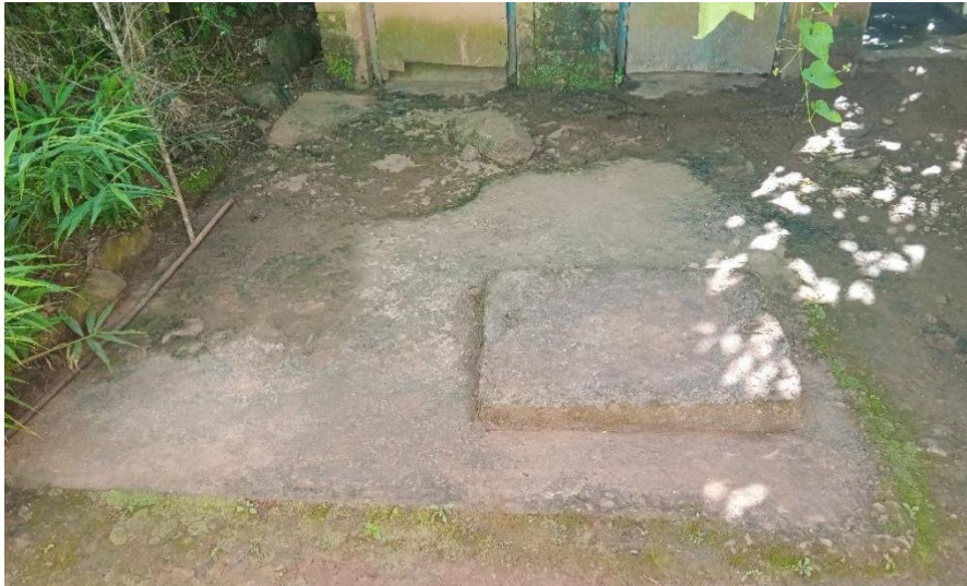
Figure 3: Fully Lined Tank.
