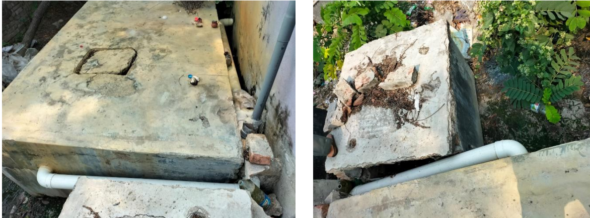
Figure 6: Containment technologies and their connections in Paikgachha Municipality. (Toilet outlets connected to open drains) (Source: Field Survey 2023/ O.CREEDS_ WaterAid Bangladesh).
