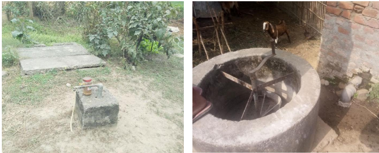
Figure 6: Types of biogas digesters in Kolhabi Municipality.
