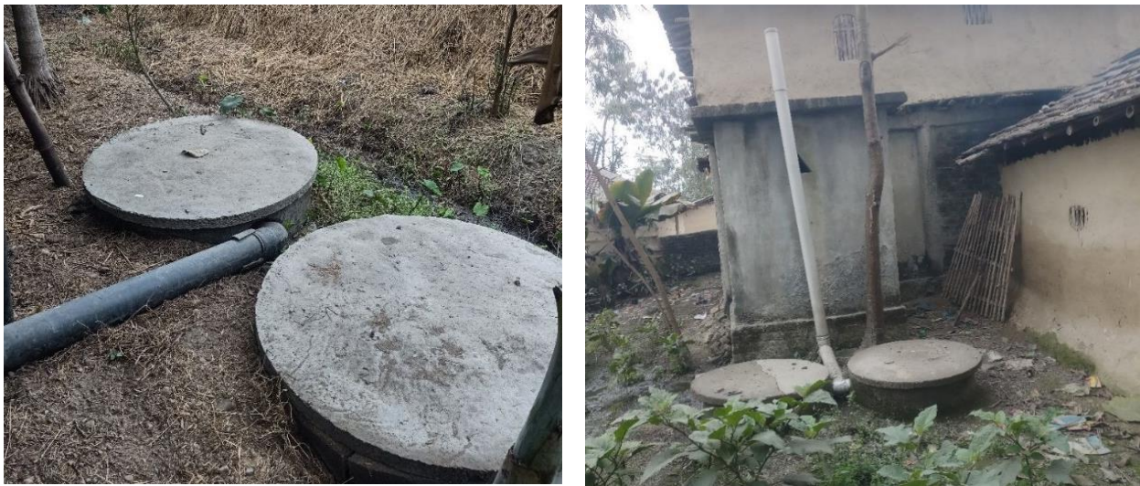
Figure 8: Inappropriate design of twin pits, the distance between two pits is less than 1.2m
