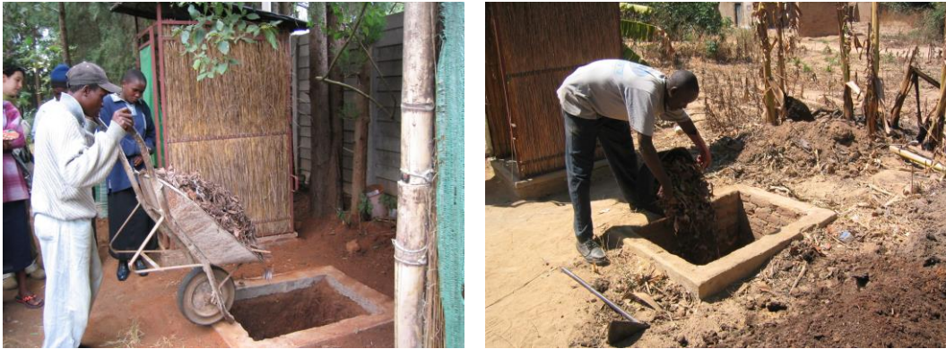
Adding leaves to Fossa alterna pits. On left at Woodhall road, on right at Epworth.
