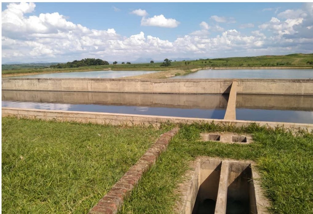
Figure 13: Kanengo Wastewater Treatment Plant- Inlet structures, Anaerobic and facultative Ponds (Mkwezalamba and Kabika, 2023).
