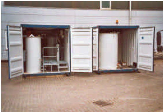
Figure 9: Waste-reuse research for simultaneous treatment of liquid, sludge and solid waste from municipalities and industries; in transportable containers, Hanau, Germany.
