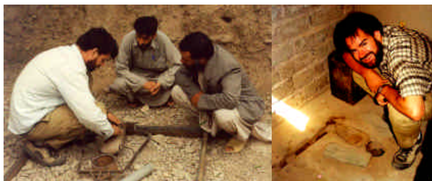
Figure 1: Moulding of slab and implemented result in Herat, Afghanistan (Photo: Dorthe Eriksson)
