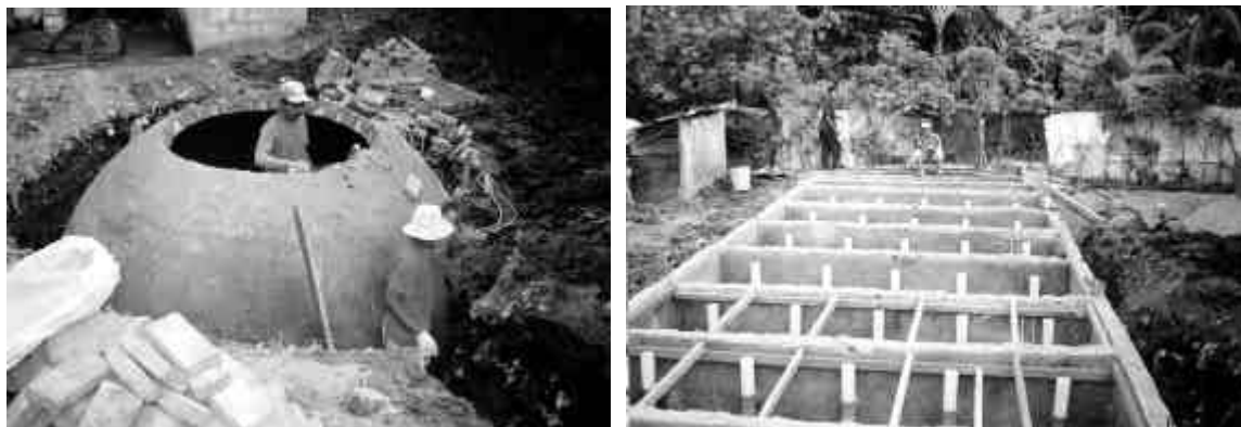
Figure 2: Biogas Digester (left) for part-stream treatment of "blackwater", brick construction with waterproof airtight plastering. Baffled reactor (right), based on anaerobic up-flow principles.
