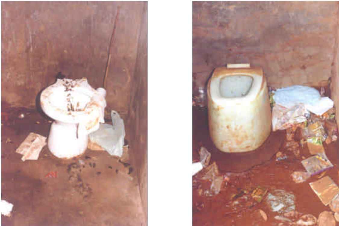
Figure 1: The existing school latrines
