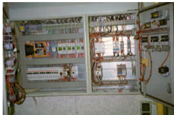
Figure 4: Recycling and energy optimisation sometimes ask for sophisticated control panels even in Ecosan projects.
