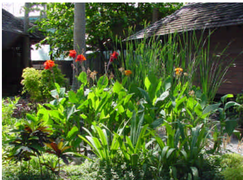
Figure 6: View of the subterra reed-bed no.4 in direct neighborhood of the bungalows
