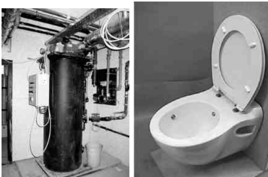
Figure 4: Vacuum pumping station (left) and vacuum-toilet of the model-house
