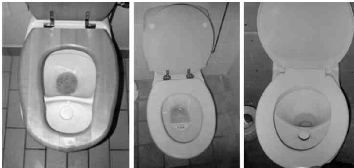
Figure 1: Separating toilets installed at the Lambertsühle, left: BB-Innovation, Sweden, centre: WostMan, Sweden, right: Roediger, Germany
