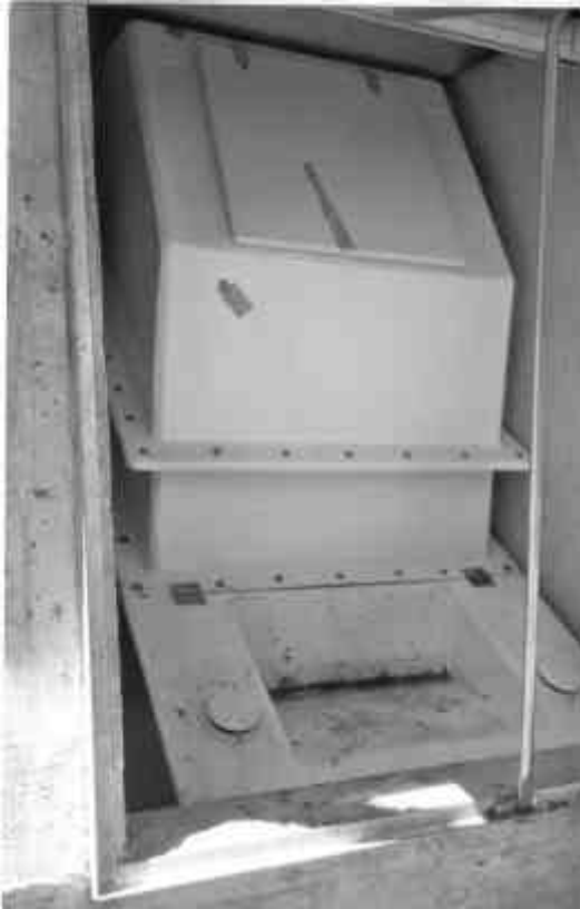
Figure 2: TerraNova composting container with improved maintenance area
