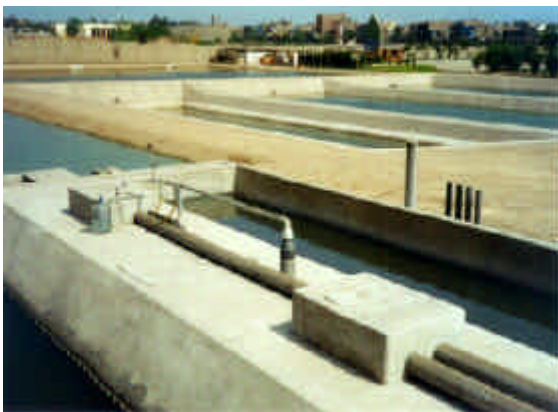
Figure 1: Appropriate decentral waste water treatment through a UASB-System in Lima.
