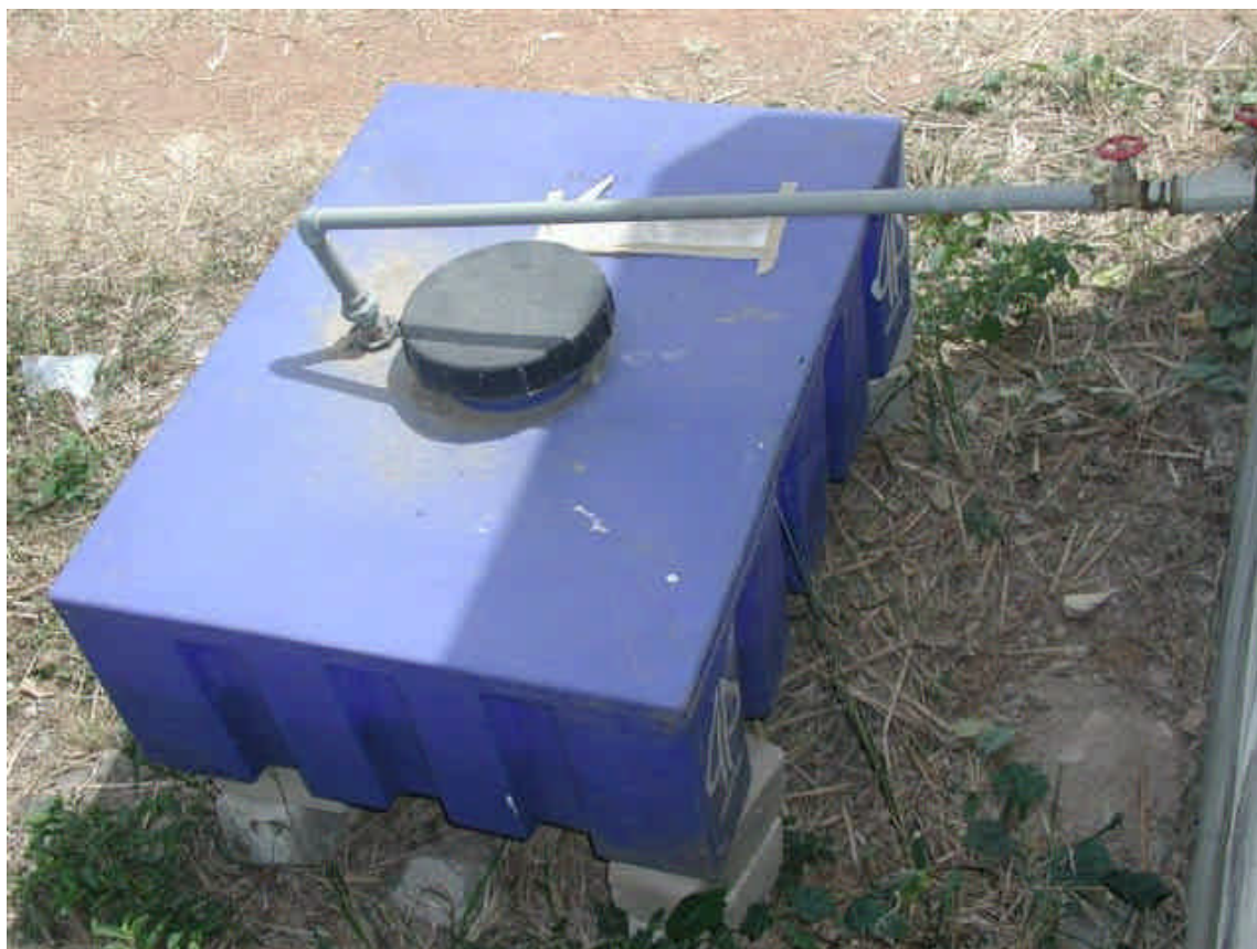
Figure 1: Urinals connected to a storage tank outside the building
