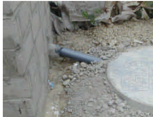
Figure 4: A short tube connects the latrine to an off set pit, which later can be connected to a small-bore sewer.
