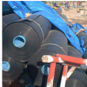
Figure 18: Bottom sealing for 6 ha landfill of integrated waste recycling and disposal plant in Chonburi, Thailand.
