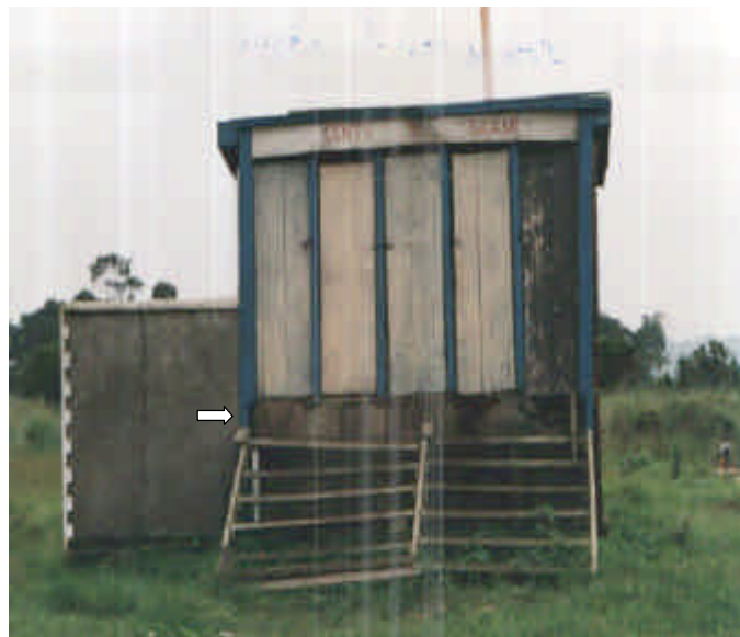
Figure 2: The old discussed VIP toilet (note the rised structure due to gro und water table).
