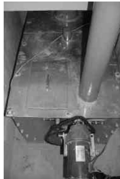
Figure 2: bio toilet treatment tank
