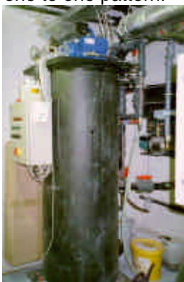
Figure 3: Vacuum-system reduces water use for Toilet Flushing in apartment building; before anaerobic treatment, Freiburg, Germany.
