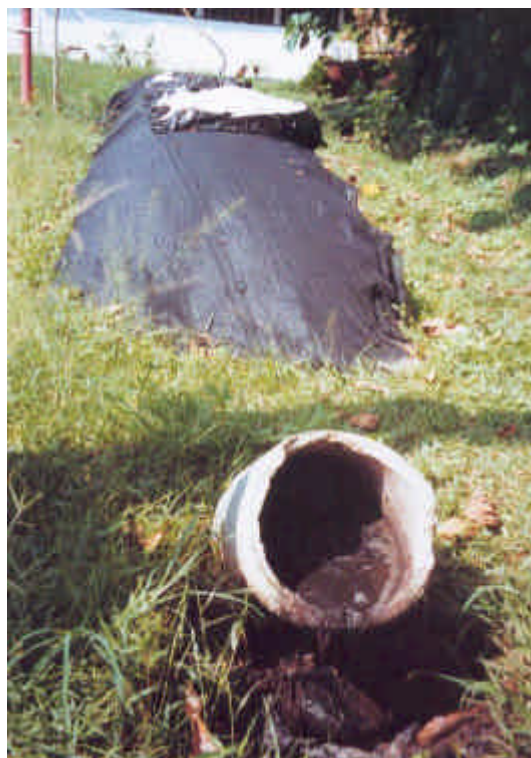
Figure 6: A common type of agricultural biogas plant in Cuba consisting of a long plastic tunnel with an in- and outlet made of concrete tubes:
