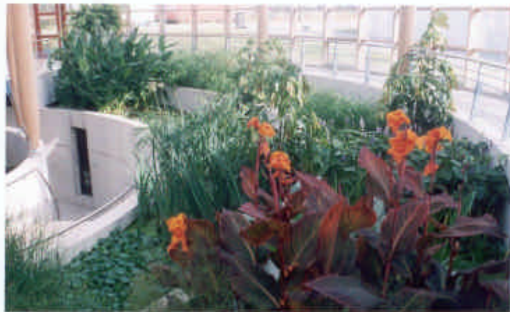
Figure 1: The “living machine” in Noorderdierenpark, treating the wastewater produced by human activities as well as the sludge produced by the membrane treatment of the hippo, sea turtle and penguin wastewater.
