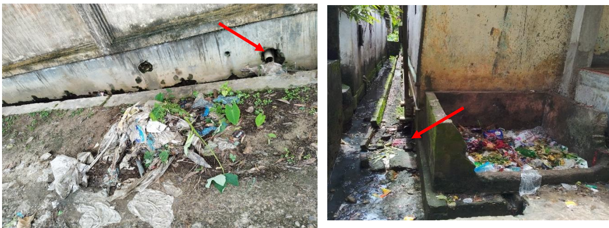
Figure 6: Containment technologies and their connections in Moulvibazar. Left: Toilet outlet pipe connected to direct drain, Right: Toilet pipe connected to open environment. (Source: Feasibility study 2020-21/DPHE).
