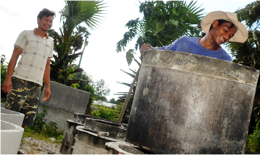
At a manufacturing site in Kampong Chhnang, Cambodia, latrine business team members produce cement rings for pits Credit: Miguel Jerónimo Photography
