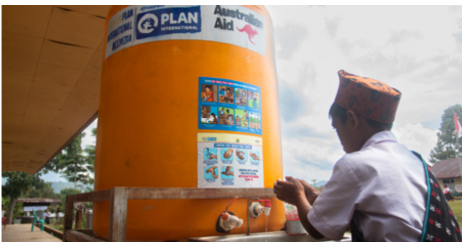
A student accesses a handwashing station installed by Yayasan Plan International Indonesia at their elementary school in East Nusa Tenggara province Credit: Yayasan Plan International Indonesia
