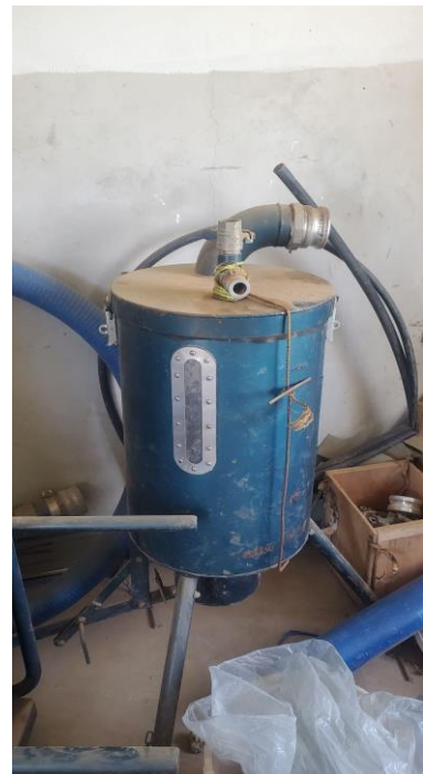
Figure 7: eVac pump used to empty pits.
