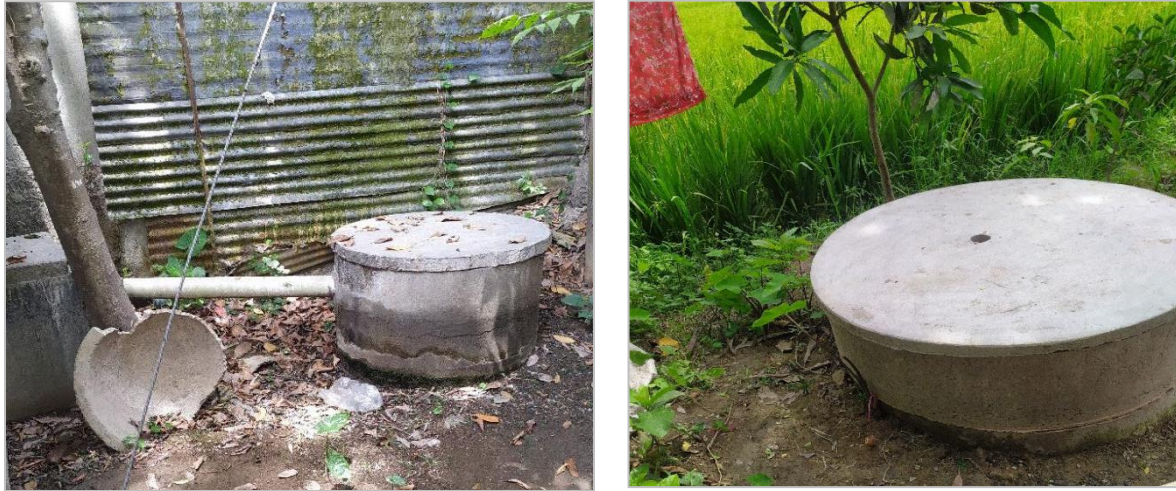
Figure 6: Containment technologies and their connections in Bera Municipality. (Source: Field Survey 2023/ O.CREEDS_ WaterAid Bangladesh).
