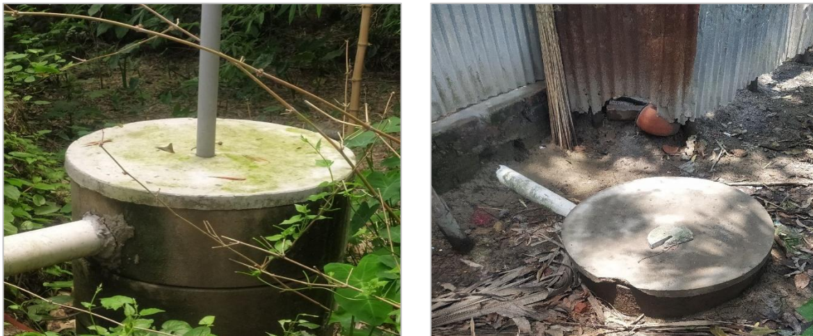
Figure 6: Containment technologies and their connections in Sreemangal Municipality (Source: Field Survey 2023/ O.CREEDS_WaterAid Bangladesh).
