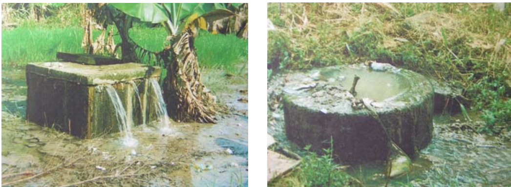
Figure 5. 10: Bleeding manholes due to blockage in parts of the FCC
