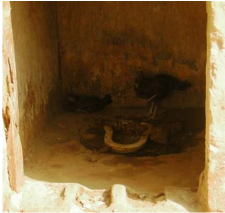
Figure 5. 21: Shared pour flush toilet in poor condition in Chika
