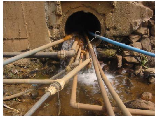
Figure 5.4: Illegal pipe connections to water mains (Krohs, 2004)
