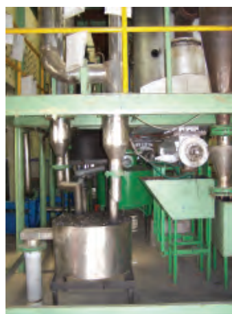
One of Desipower biomass plants
