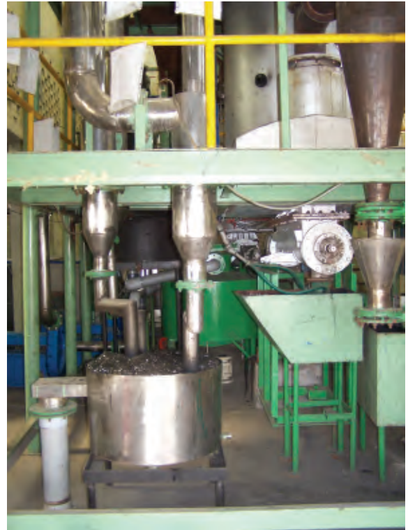
Figure 17 A biogas digester plant
