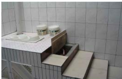
Figure 5: Open hatch shows access to the urine pipe and urine storage tank of the UDD squatting toilet (source: Plan China)
