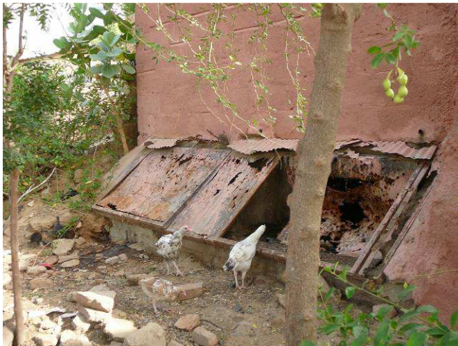
Fig. 9: Rusted iron covers of faeces chambers are falling apart, - no more drying of faeces is therefore possible (source: Stefan Hofstetter, March 2009).
