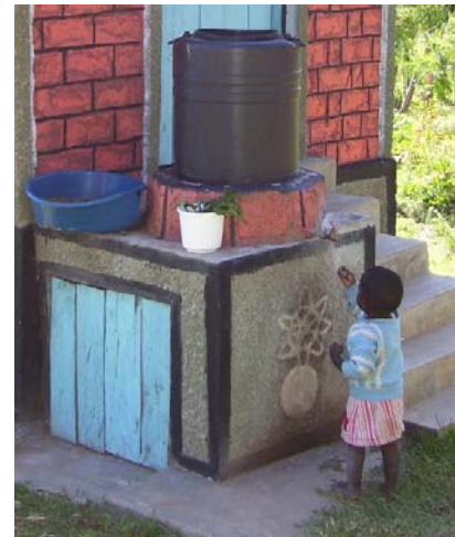
Fig. 12: Hand wash facility with 100 litre tank and tap secured in concrete located on top of urine tank storage vault (Source: Moses Wakala, GTZ-Kenya, Jan. 2010).
