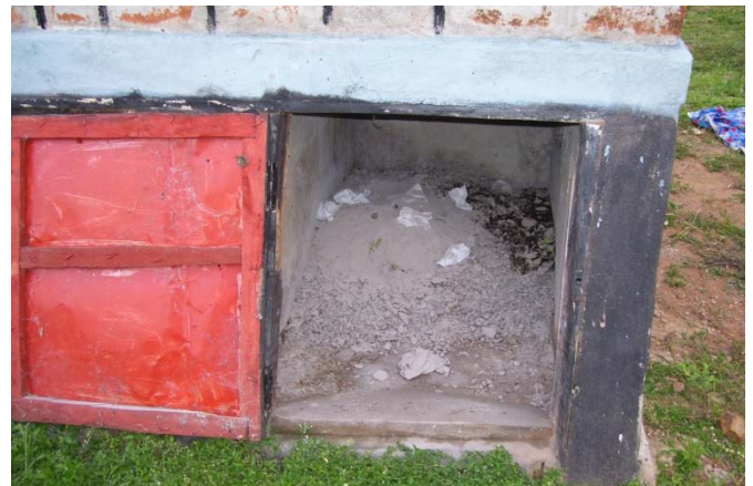
Fig. 7: Faeces collection vault which is half full (source: David Watako, GTZ-Kenya, July 2009). Note: Sufficient use of ash and appropriate use results in a dry and odour free condition of the vault.
