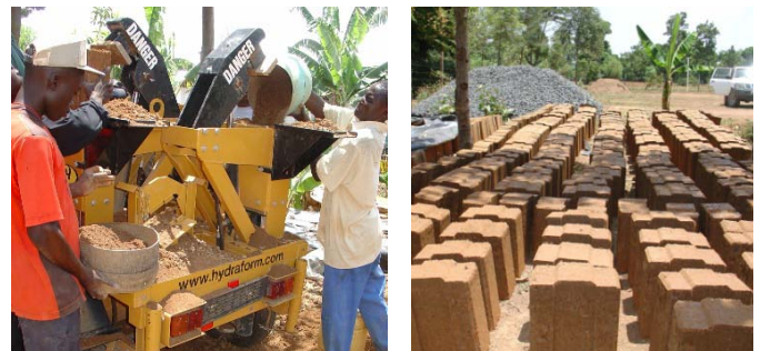
Fig. 14: Left: Production of hydraform blocks; Right: completed hydraform blocks (Source: Paul Mboya, June 2009).
